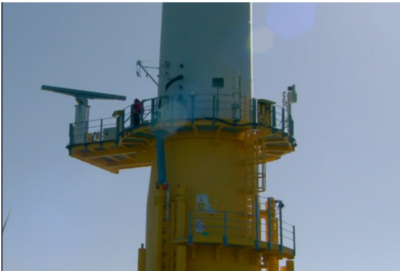
Figure 1. SCANTER 5000 radar installed on the laydown area of the work platform of turbine G01 at Thanet Offshore Wind Farm.
